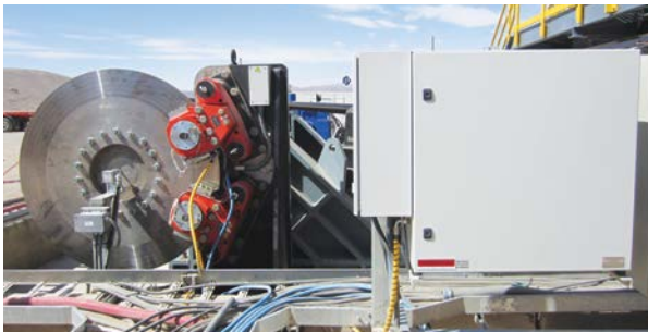
A complete Svendborg engineered brake system package, installed on a copper mine conveyor, consists of two BSFH 520 caliper brakes (red) and disc, a hydraulic power unit and a soft braking control (housed in two adjacent gray boxes on right).
